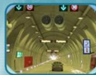
Tunnel Management System
